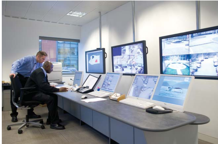
A Siemens control room
